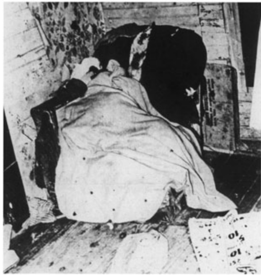
PEELING WALLS AND BARE FLOORS
