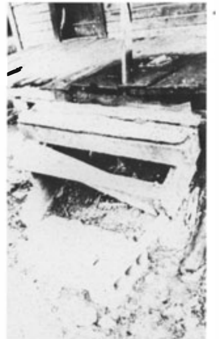
CRUMBLING FRONT PORCH
