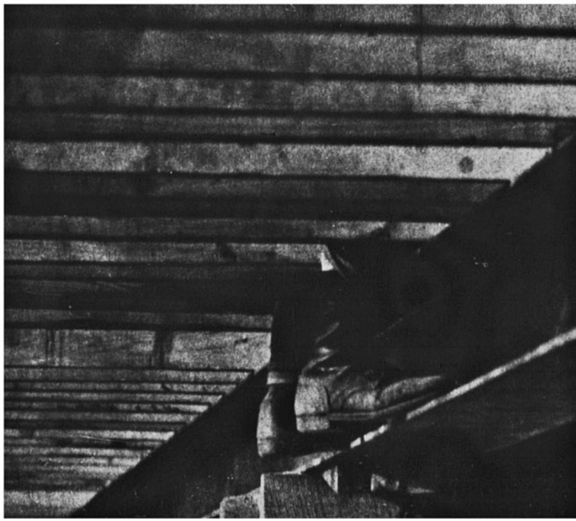
PHOTO EDITOR JAMES H. PEPLER WAS LET LOOSE AT THE CONSTRUCTION SITE OF THE INTERSTATE HIGHWAY THROUGH MONTGOMERY, AND THIS IS WHAT HE FOUND UNDER A NEW BRIDGE.
