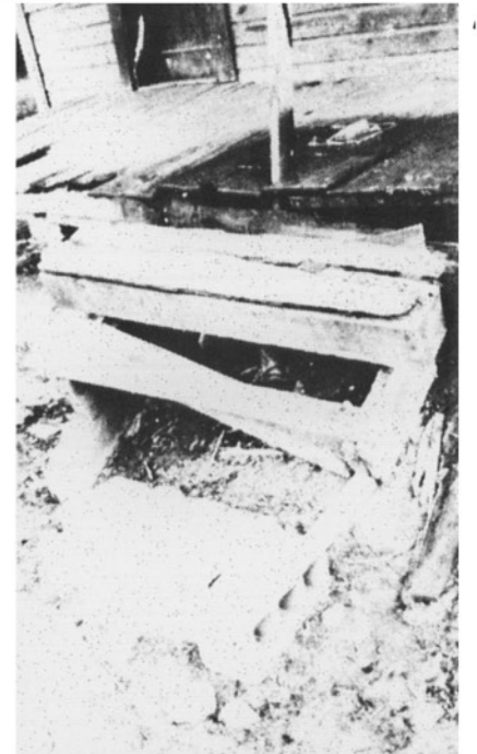
CRUMBLING FRONT PORCH
